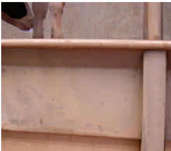
Initial hard deposits on the wall forms within a few days.
