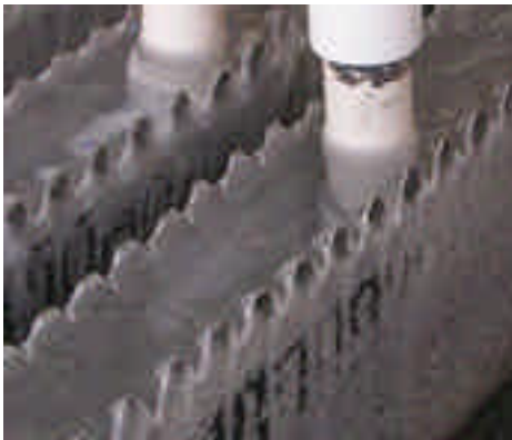
Initial hard deposits on plate ice machine forms within a few days, has to be cleaned with acid.
