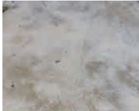
Before treatment, scale deposits formed on the floors and surrounding area.
